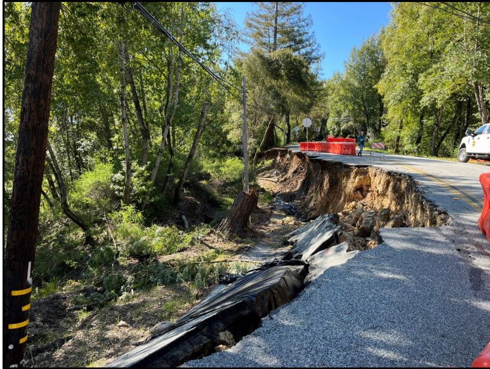
Figure B.2. A washed-out road (due to heavy rain and snow storms) within a residential community.
